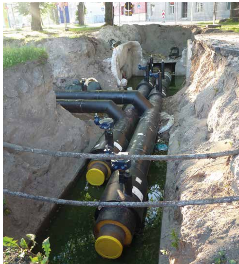
Installation of heat network pipe in Tallinn, Estonia (Dmitry G, Wikimedia Commons)
