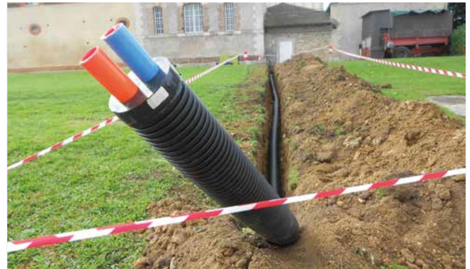
Expansion bend in the Roeselare heat network
