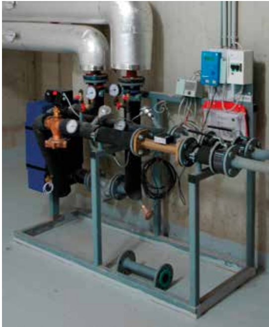
Apartment building substation, power 300 kW, dimensions 1 x 0.5 x 1 m (Danfoss)
