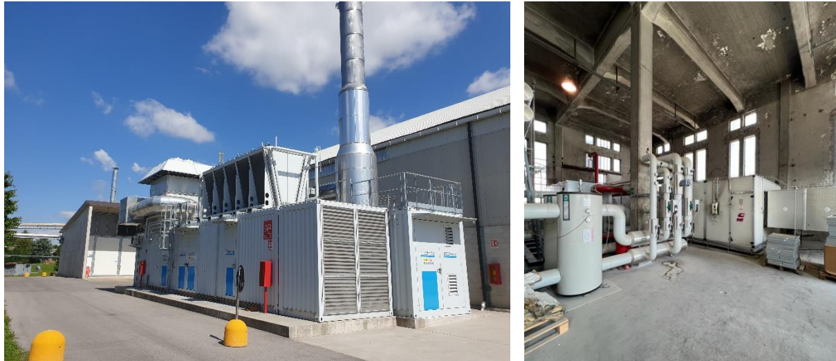
Figure 5: CAMA Papermill and Cogenerator Plant (CHP)
